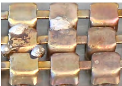
2 Too high temperature
